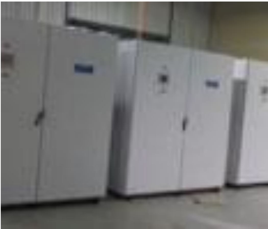
Three of our 100kW Special-Application Transmitters on the Shop Floor
